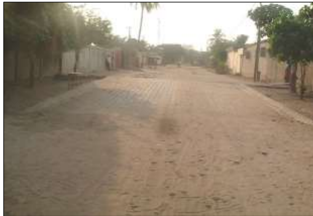
Figure 9. Work after 15 years of exploitation (2018)
